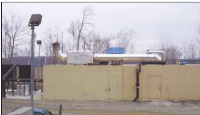
The Okemo Mountain Resort constructed a separate building (entered through doorway at left) to house the Miratech SCR system reactant storage tank, injection panel and all other components, next to the Cat 3516B engine-IR Centac compressor package enclosure (entered through doorway at right).
