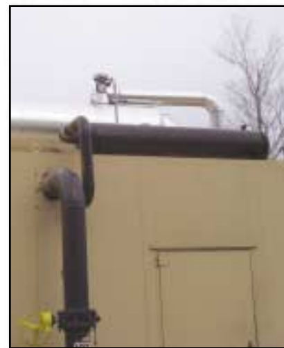
A closeup view of the urea injector wand location in the exhaust pipe. The exhaust piping was insulated to maintain exhaust temperatures for the catalytic reactions, and a straight run of pipe was necessary for proper mixing and urea hydrolysis.
