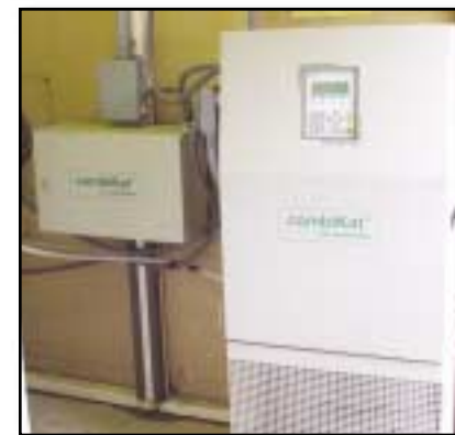
The urea injection panel is a prepackaged unit containing the urea pump, air compressor and PLC for the proper metering of the aqueous urea reductant. Miratech sells, specifies and supports SCR catalytic systems from the Swiss company HUG Engineering.
